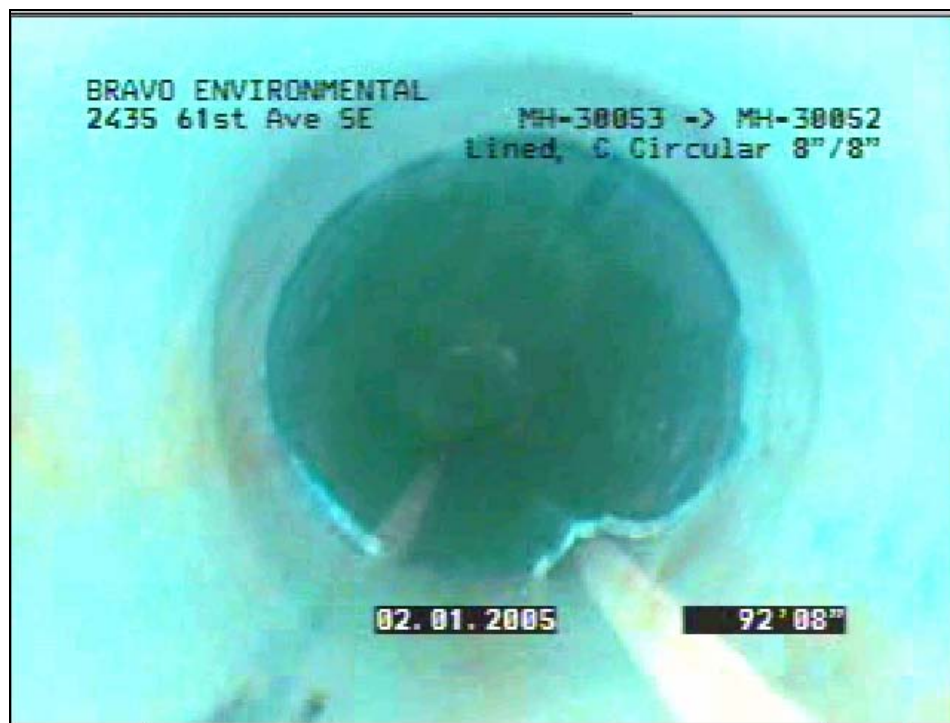
Figure 9 – Curled edge on the upstream edge of a CIPP spot repair in Mercer Island
