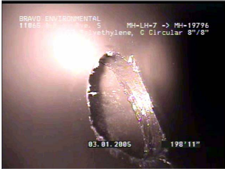
Figure 5 – Black HDPE pipe in Skyway
