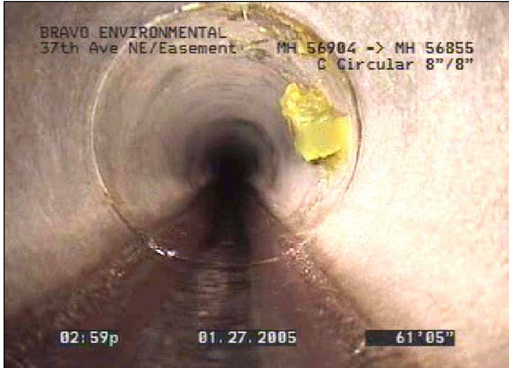
Figure 10 – Photo of pipe in Lake Forest Park Remnants of grout remain inside the pipe after grouting the joint.
