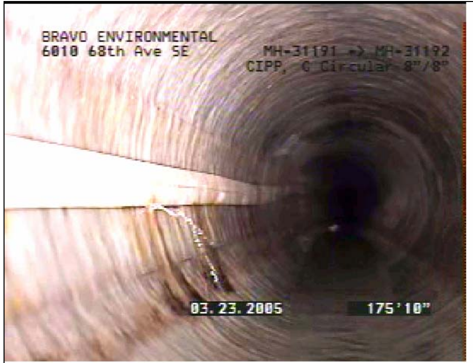
Figure 8 – Active leak through CIP liner in Mercer Island
