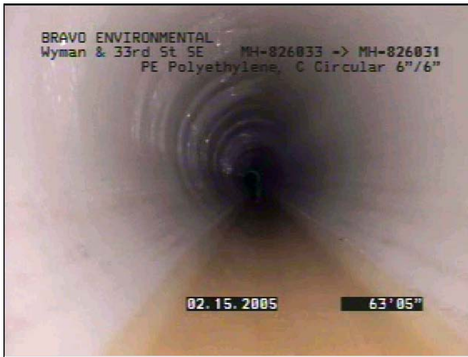
Figure 6 – Gray HDPE pipe in Auburn
