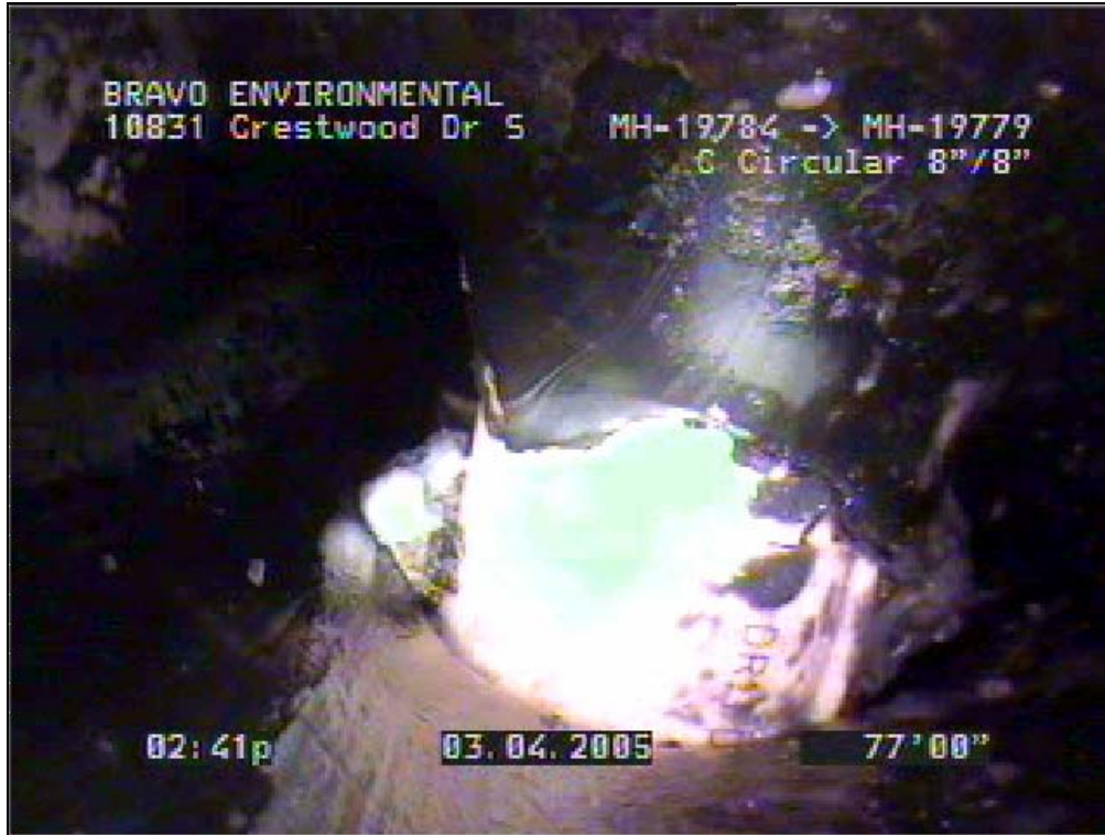
Figure 2 – Irrigation pipe bored through a side sewer in Skyway
