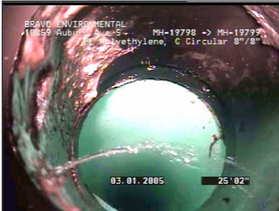
Figure 3 – Leak at the bottom of a welded saddle connection in Skyway Picture was taken looking up the lateral from inside the sewer main.
