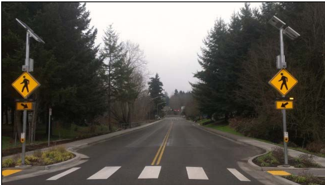
Figure 1.27: Application of RRFBs in Mountlake Terrace, Washington
