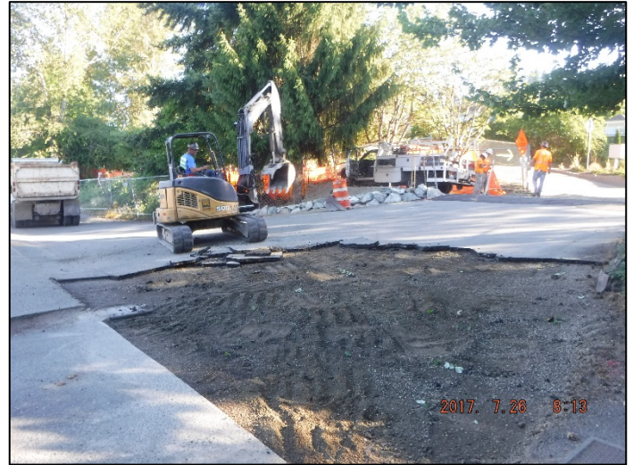
Asphalt removal and installation of CSBC in preparation of asphalt paving of driveway 6 approaches
