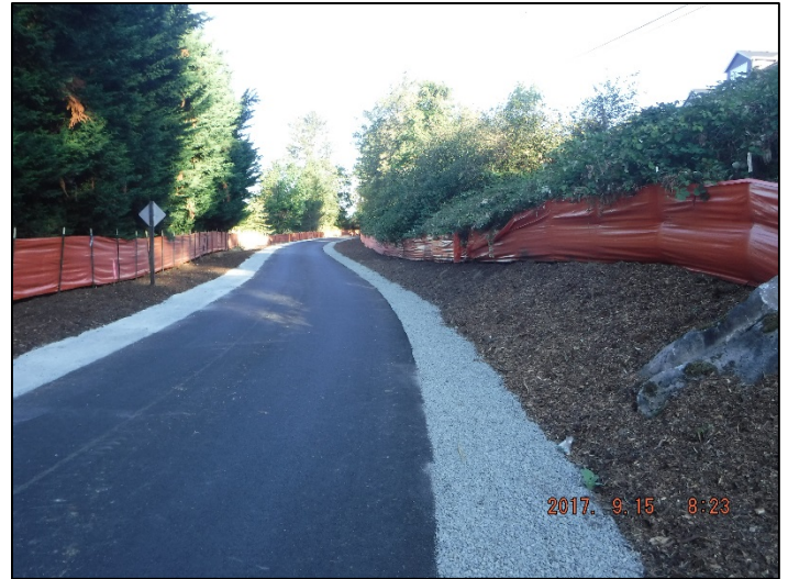
Completed installation of wood chip mulch on the edges of the trail.
