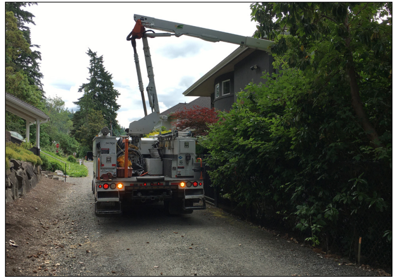
Preconstruction activities also include relocating utilities to make room for a wider trail.
