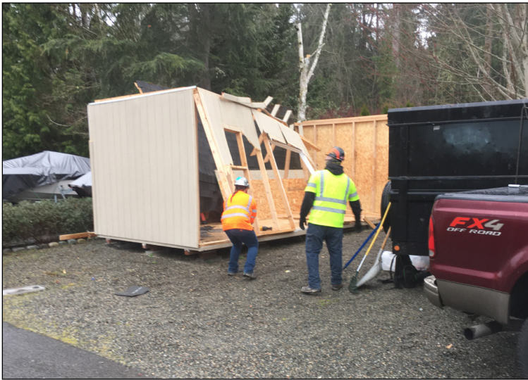
Removing encroaching structures inside the trail construction boundaries, in preparation for trail construction.
